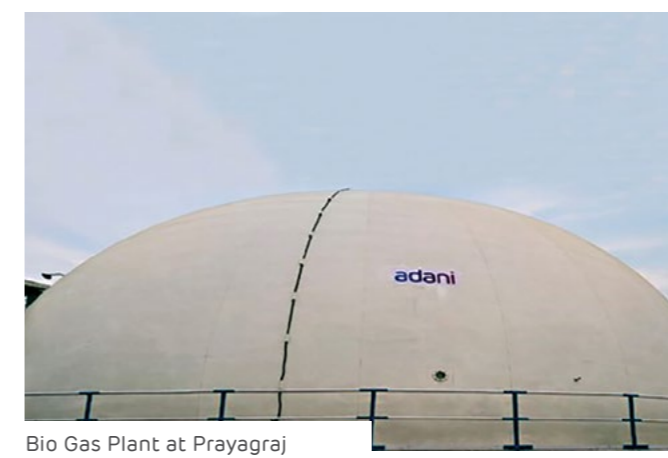
Bio Gas Plant at Prayagraj
