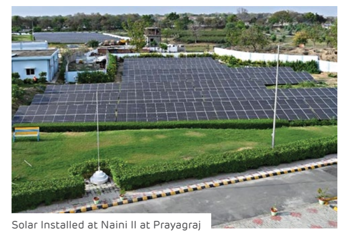
Solar Installed at Naini II at Prayagraj
